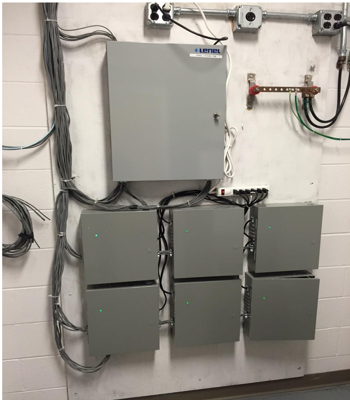
Panel with Power Supply
