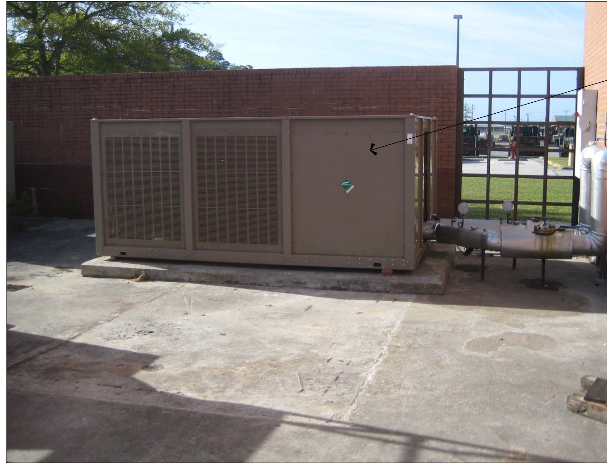
1 EXISTING 60 TON CHILLER TO BE REMOVED AT, BLDG. 4401 W-302 W-302 NO TO SCALE
