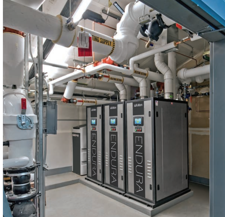
▶ Three Endura boilers are integrated directly into a primary-only variable flow installation to provide building heat.
